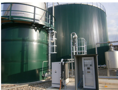
Complete System configured with Process Connection, Sample Line & Analyzer
